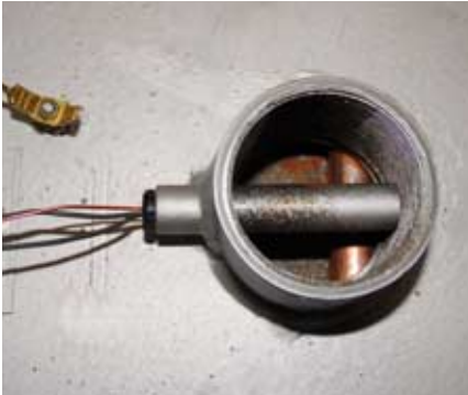
sensor of the safety temperature limiter STB in the boiler flow line
