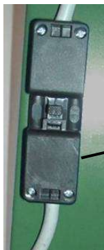
Connector on the boiler
